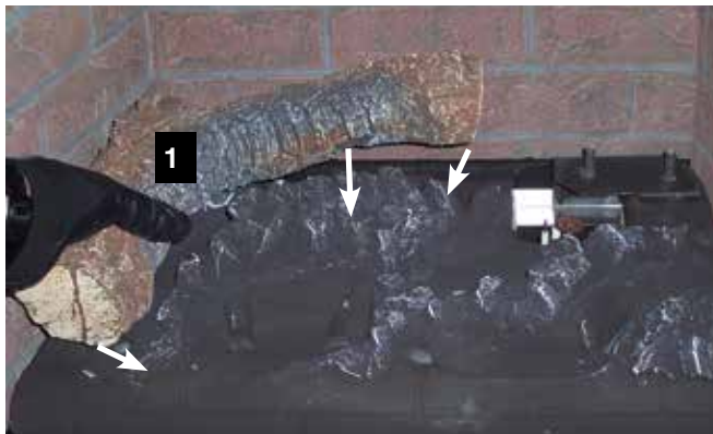
Log 1 location on burner
